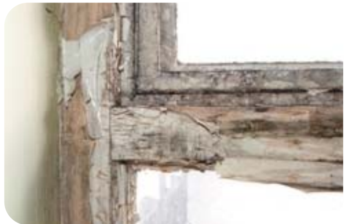
e.g. damage to a window frame
