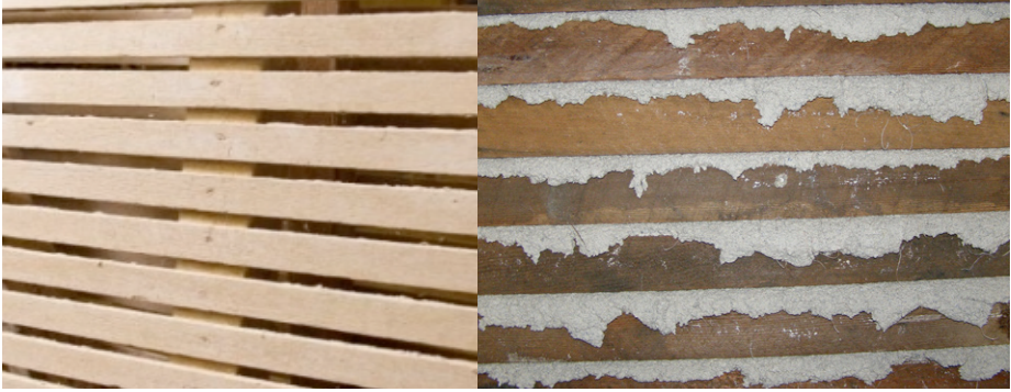
Laths fixed ready for plaster and nibs, hooking over the laths holding the plaster in place
