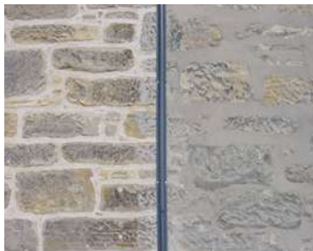
Good pointing against poor pointing
